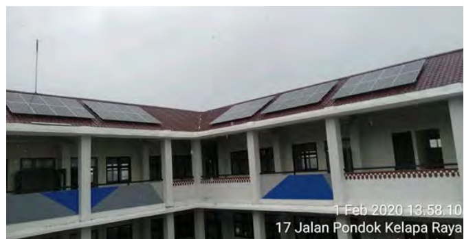
Gambar 2.4 Pemasangan Solar Panel Frame di atap SMKN 69 Jakarta Timur Picture 2.4 Installation Frame Solar Panel on the roof SMKN 69 East Jakarta
