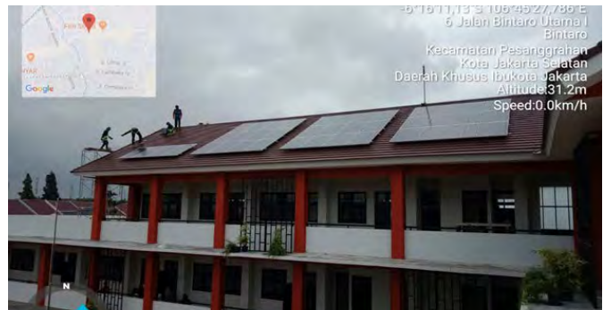
Gambar 2.2 Pemasangan Solar Panel Frame di atap SDN 04 Bintaro Pagi Picture 2.2 Installation Frame Solar Panel on the roof SDN 04 Bintaro Pagi
