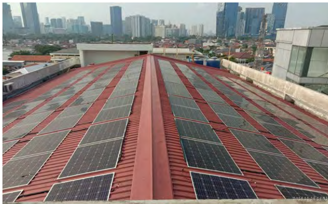
Gambar 1.1 Pemasangan Solar Panel J-Leaf di atap Gedung B ESDM Minerba Picture 1.1 Installation of J-Leaf Solar Panel on the roof of ESDM Minerba Building B
