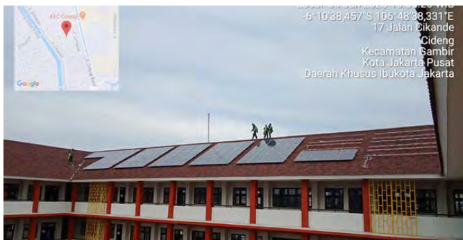
Gambar 2.1 Pemasangan Solar Panel Frame di atap SDN Cideng 04 Picture 2.1 Installation Frame Solar Panel on the roof SDN Cideng 04
