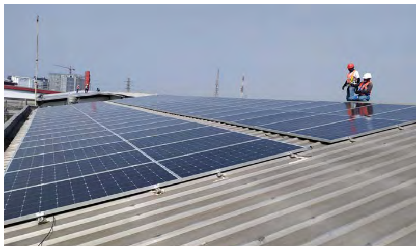
Gambar 1.3 Pemasangan Solar Panel Frame di atap Pabrik Toyota Astra Motor Picture 1.3 Installation Frame Solar Panel on the roof Toyota Astra Motor Factory
