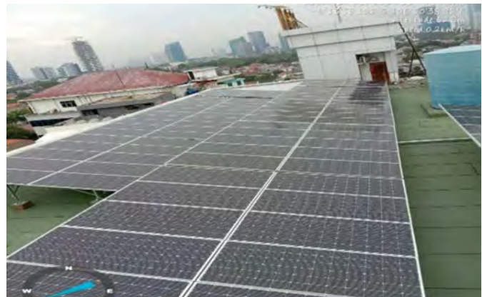
Gambar 1.2 Pemasangan Solar Panel Frame di atap Gedung C ESDM Minerba Picture 1.2 Installation of Framed Solar Panel on the roof C of ESDM Minerba Building
